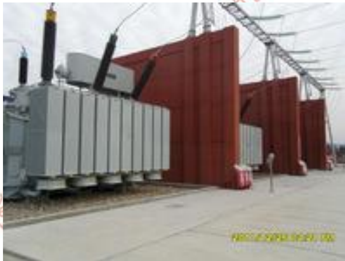
220 Kv impedance matching power transformer
